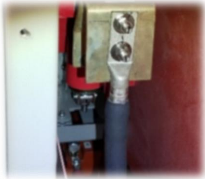
Figure 16: Power Source Cable Connection
