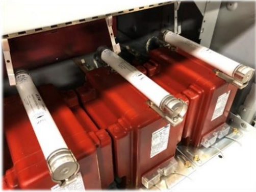
Figure 6: Fixed Mount Wye Configuration Voltage Transformers (PTs)*
