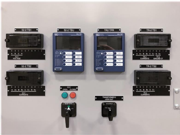
Figure 4: ANSI/IEEE 1547 Utility Intertie Protection with Redundant Relays, Test Switches, Pistol Grip CB Switch & (86) Knob Grip
