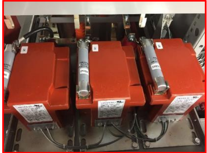
Figure 8: 15kV – Bottom Drawer Mounted Voltage Transformers (PTs) & Draw-out Access to Primary Fuses*
